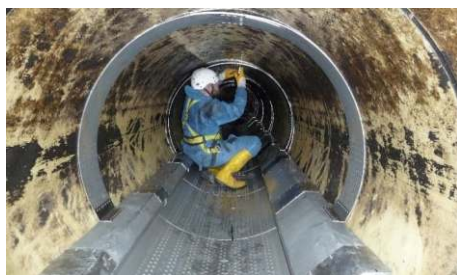
(a) Riothermie Rotterdam
